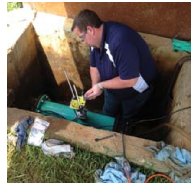
Figure 2: The FPI Mag™ Flow Meter Installation
