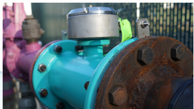
An electromagnetic meter installed in a pipeline
